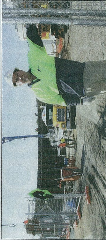
WORKS UNDERWAY... Pictured, Ausform Site Supervisor, Brian Fitzgerald in front of the extensive works underway at Goulburn Valley Water in Numurkah. Photo: Julie Moore.
